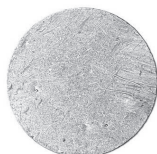
10c, T1 damaged clad
